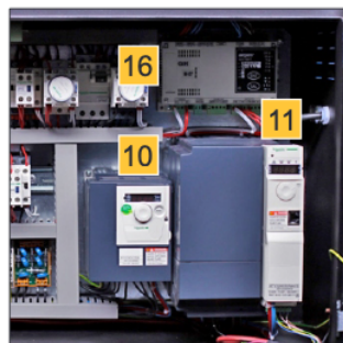
17 Hoist electric cabinet
