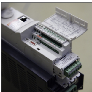
11 Hoist Frequency inverter
