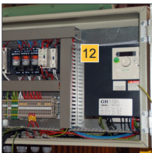
9 Crane control panel
