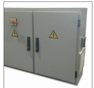
9 Crane control panel
